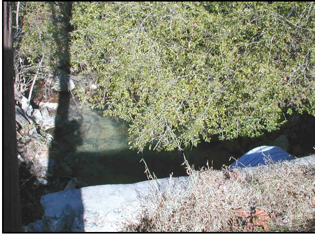
One of the branches of Falling Creek disappears into a culvert under 12 th Avenue NE.
