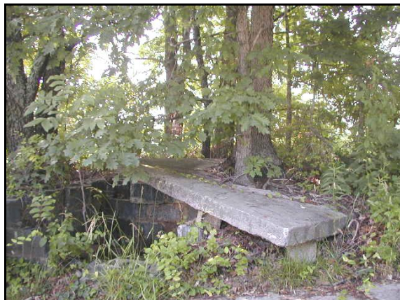
A close look at this abandoned water tap on 9 th Street Drive NE shows a tree growing through the manhole cover.
