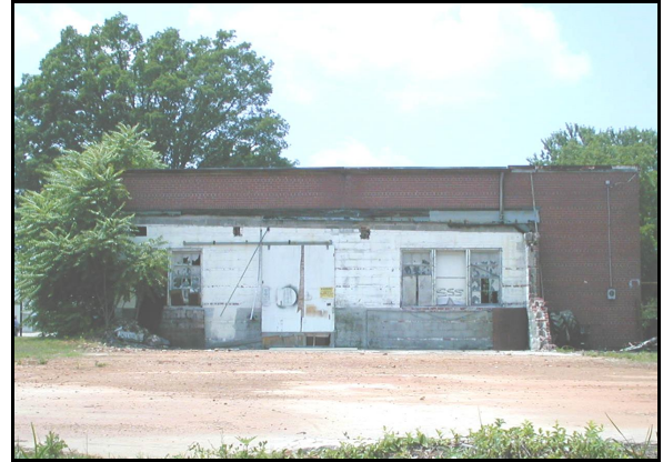
The former service station on the corner of Highland Avenue NE and 12 th Street NE is marked with graffiti and broken windows.
