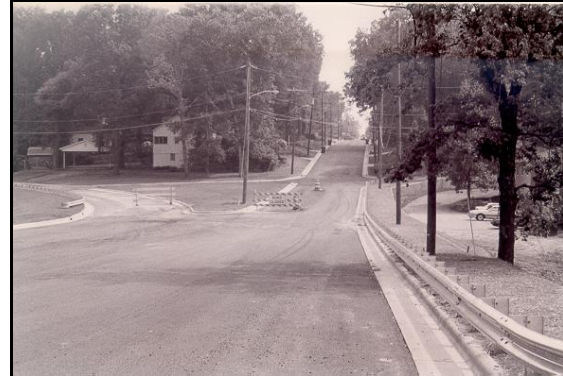
Construction of the one-way pairs, 8 th Street NE and 9 th Street NE at 13 th Avenue NE in 1998.
