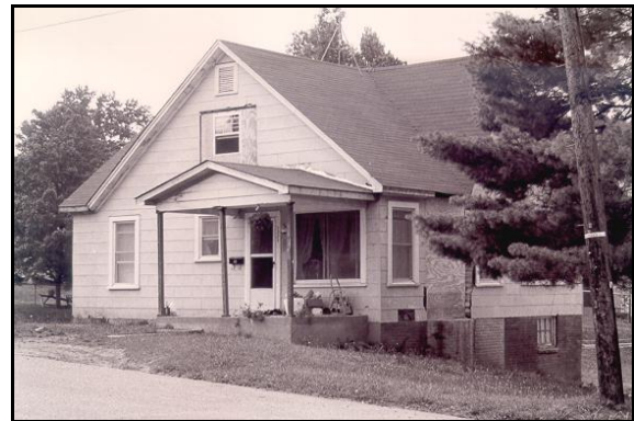
This house on 13 th Avenue NE remained an eyesore for several years because the owners lived out of the state and let it fall into disrepair.
