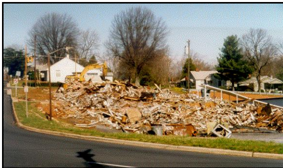
The Baker Heritage building on 9 th Avenue NE was vacated and demolished in March 1998.
