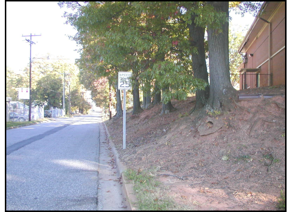
The bank at Highland Recreation Center is eroded to the point that tree roots are exposed.
