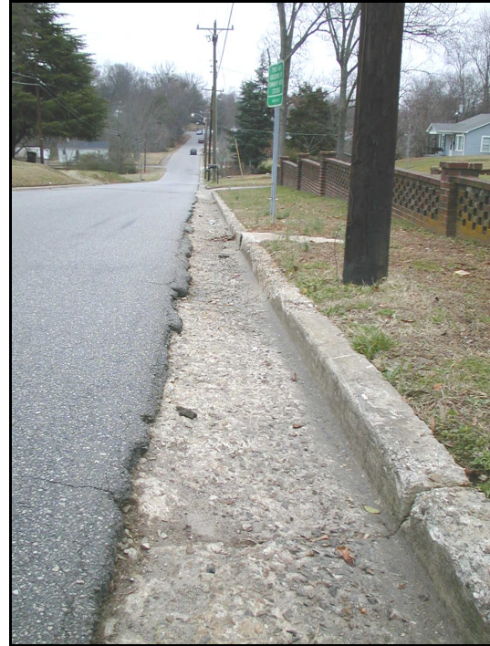
Crumbling curb on 12 th Avenue NE contributes to the neglected appearance of the neighborhood.
